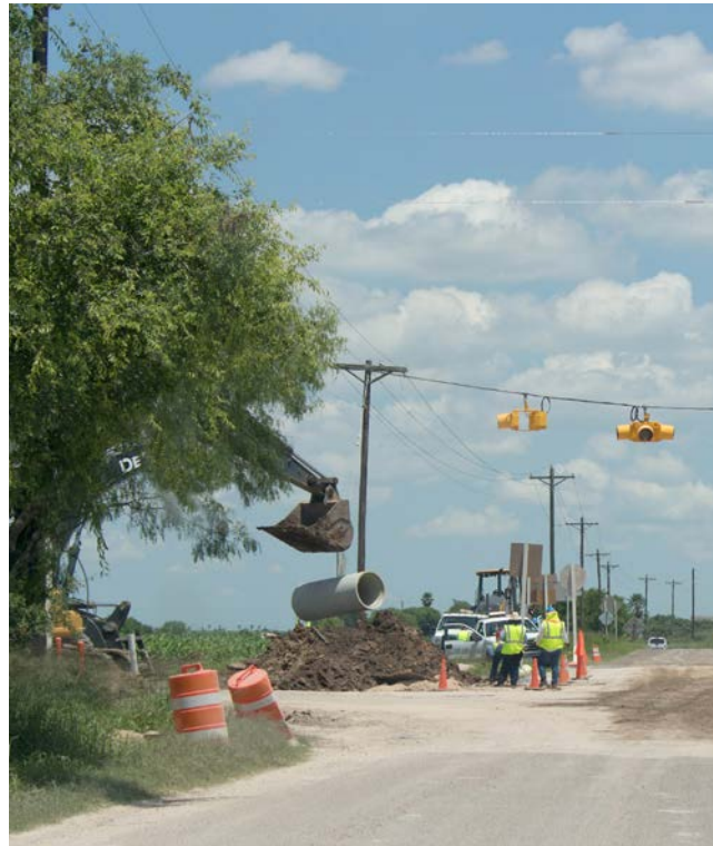
IMAGE: Drainage system installed in Weslaco near, but not in, colonias (Credit: Danielle Rivera, April 2015).
