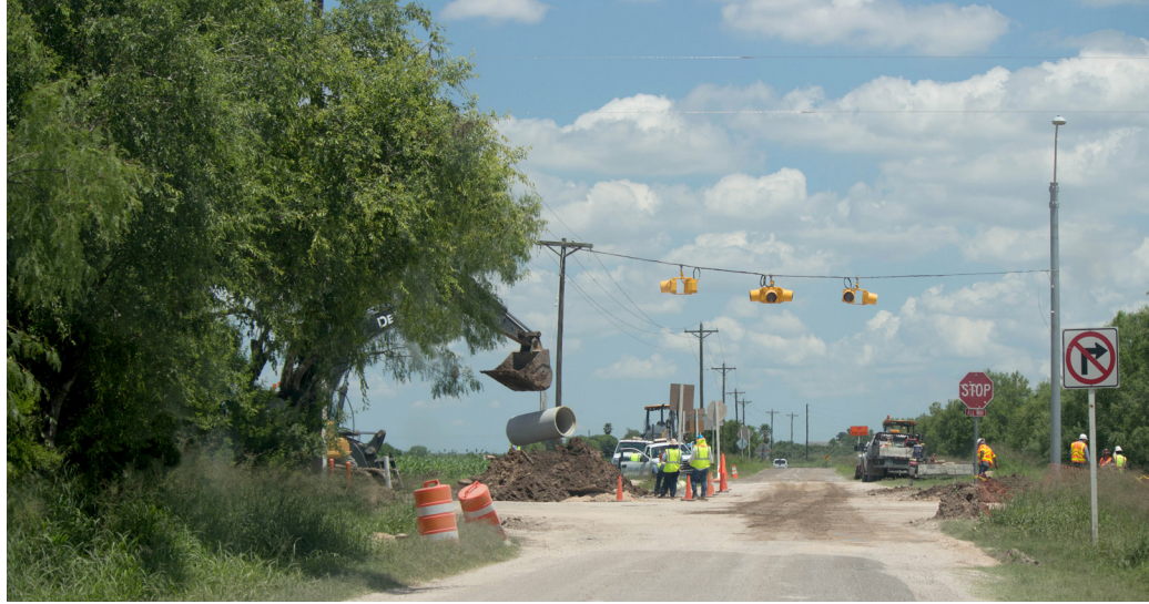
Stormwater management drains being installed at an intersection outside of Weslaco, Texas. Source: Danielle Zoe Rivera.
